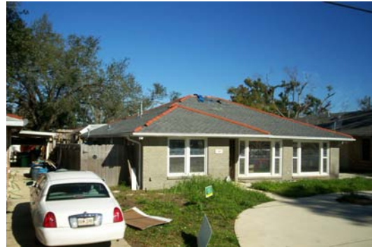
But people are trying to get their lives back together. This house had a hole in the roof where the people living there had to climb on top to get out. Now they are working on rebuilding.
